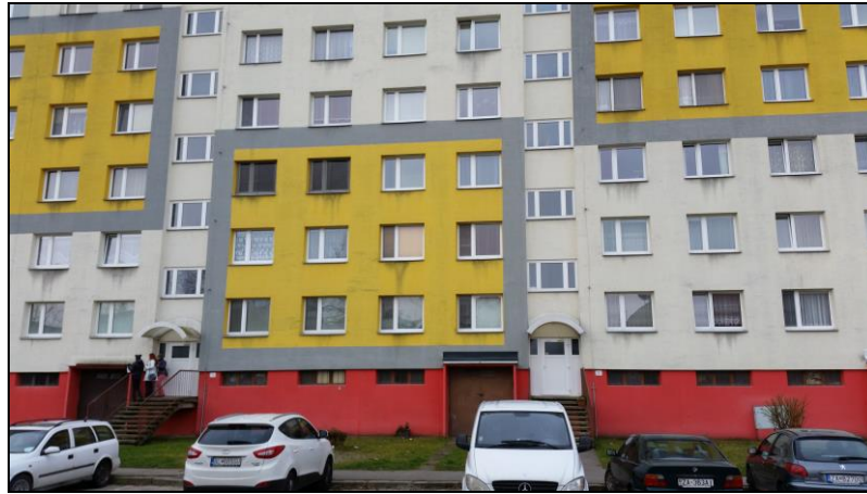
Fig.2: North facade – local contamination show process of water run-off from sill or thermal bridges in window to sill joints. (Antošová)
