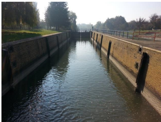
Fig. 5: Navigation lock in Itebej
