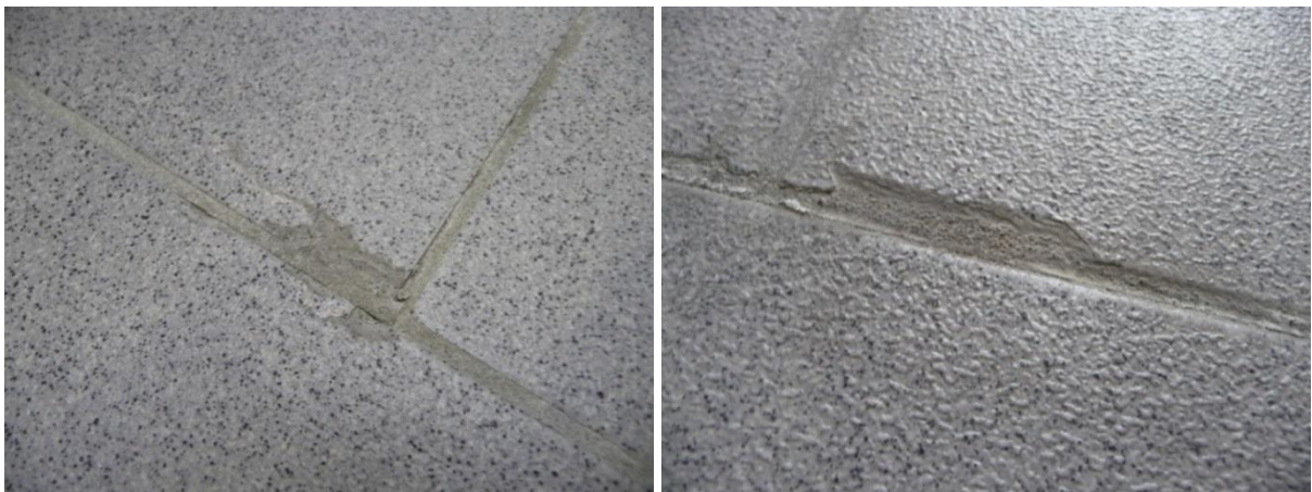
Fig. 1: Typical damage of ceramic tiles in the new floor
