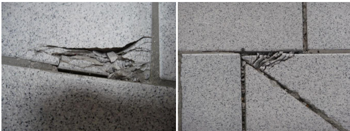
Fig. 2: Typical damage of ceramic tiles in the old floor
