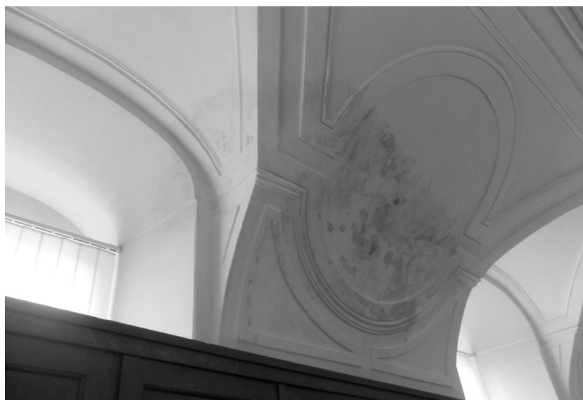
Fig. 4) Damage to part of vault situated over graphics storeroom.
