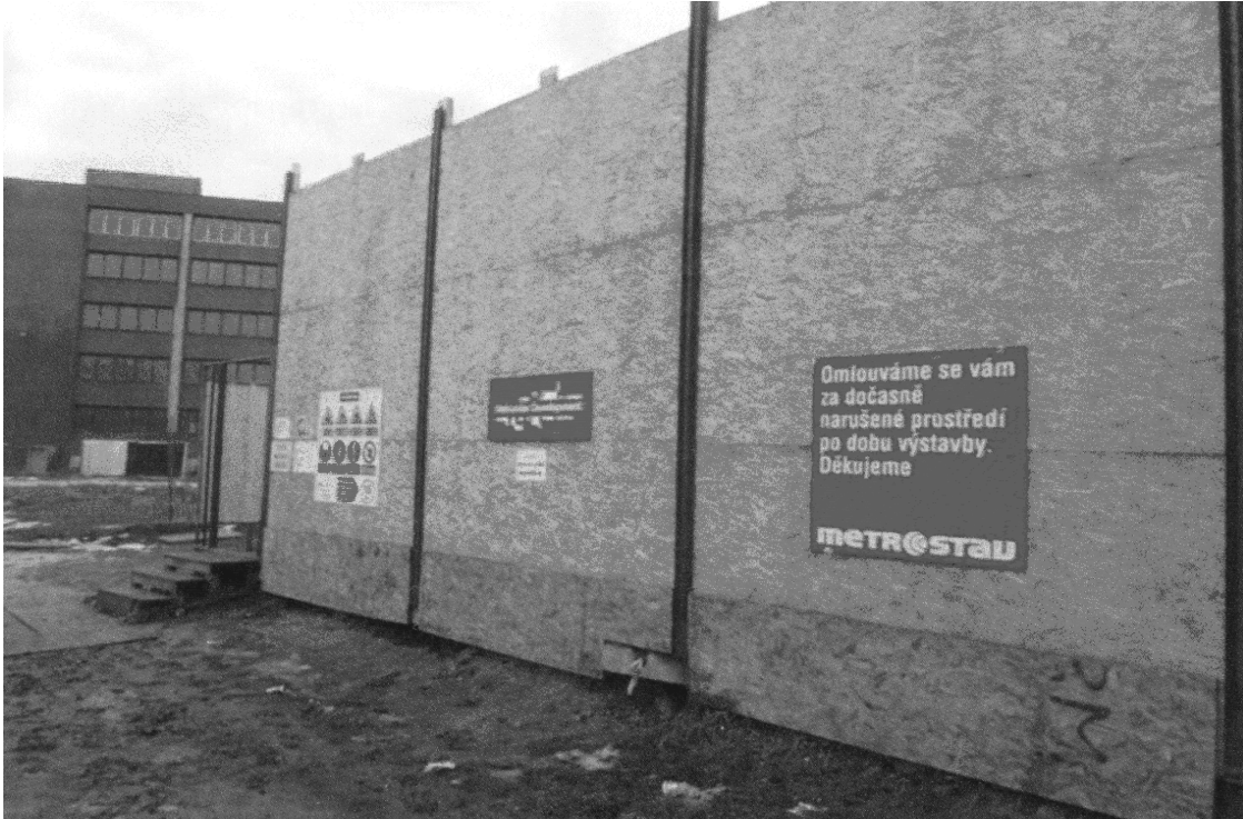
Fig. 1) Noise barrier as a specific part of the fence of a construction site
