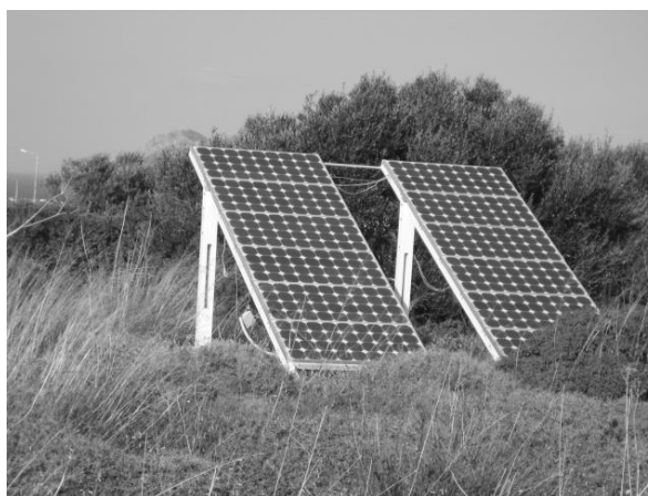
Fig. 3) Photovoltaic panels installed on a Campus expanse
