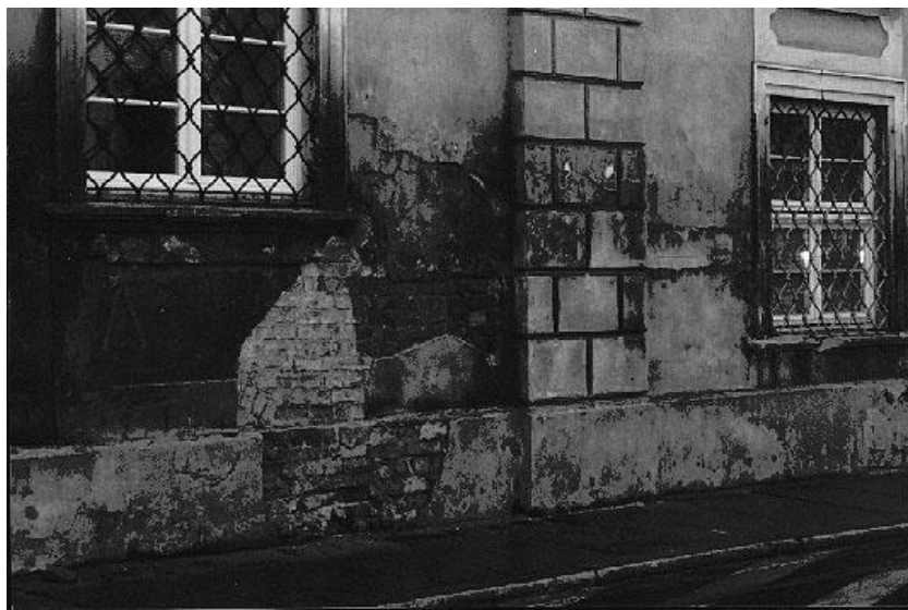
Fig. 3) Damage caused by excessive accumulation of moisture in building's west wall.
