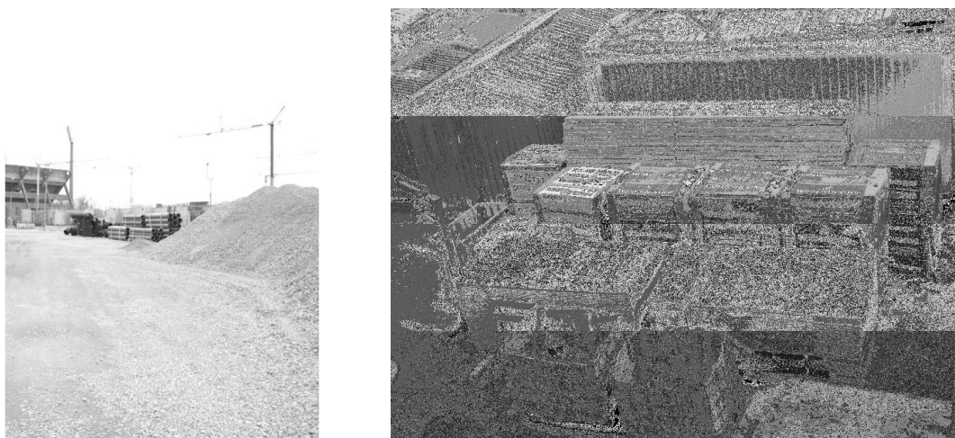
Fig. 2) Material storage at the construction site (sports hall construction in Osijek City Garden).
