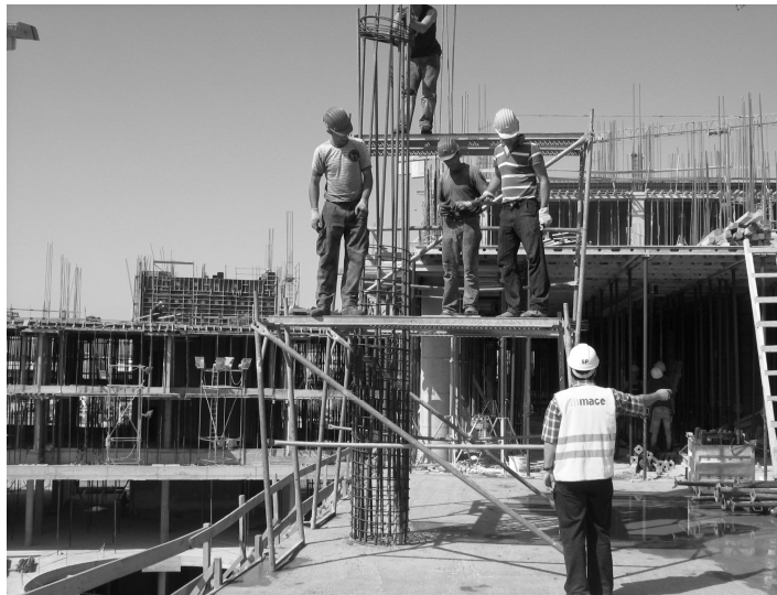
Fig. 2) Improperly made scaffoldings
